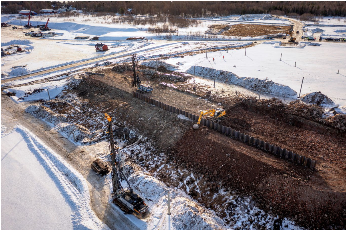
Overview of ongoing land construction works for the construction of Cinis Fertilizer's production facility in Köpmanholmen, Örnsköldsvik. Photo: Leif Wikberg
